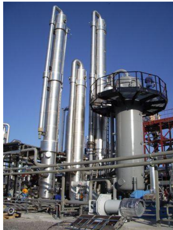
2000 nm 3 /h plant in France, 2006, 100 hours
